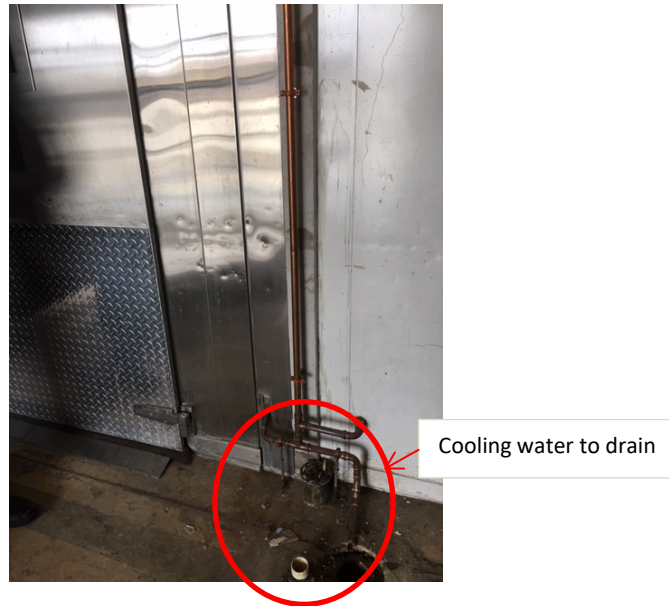
(a) Once-Through Cooled Bio-Hazardous Fridge Compressor (Before)
